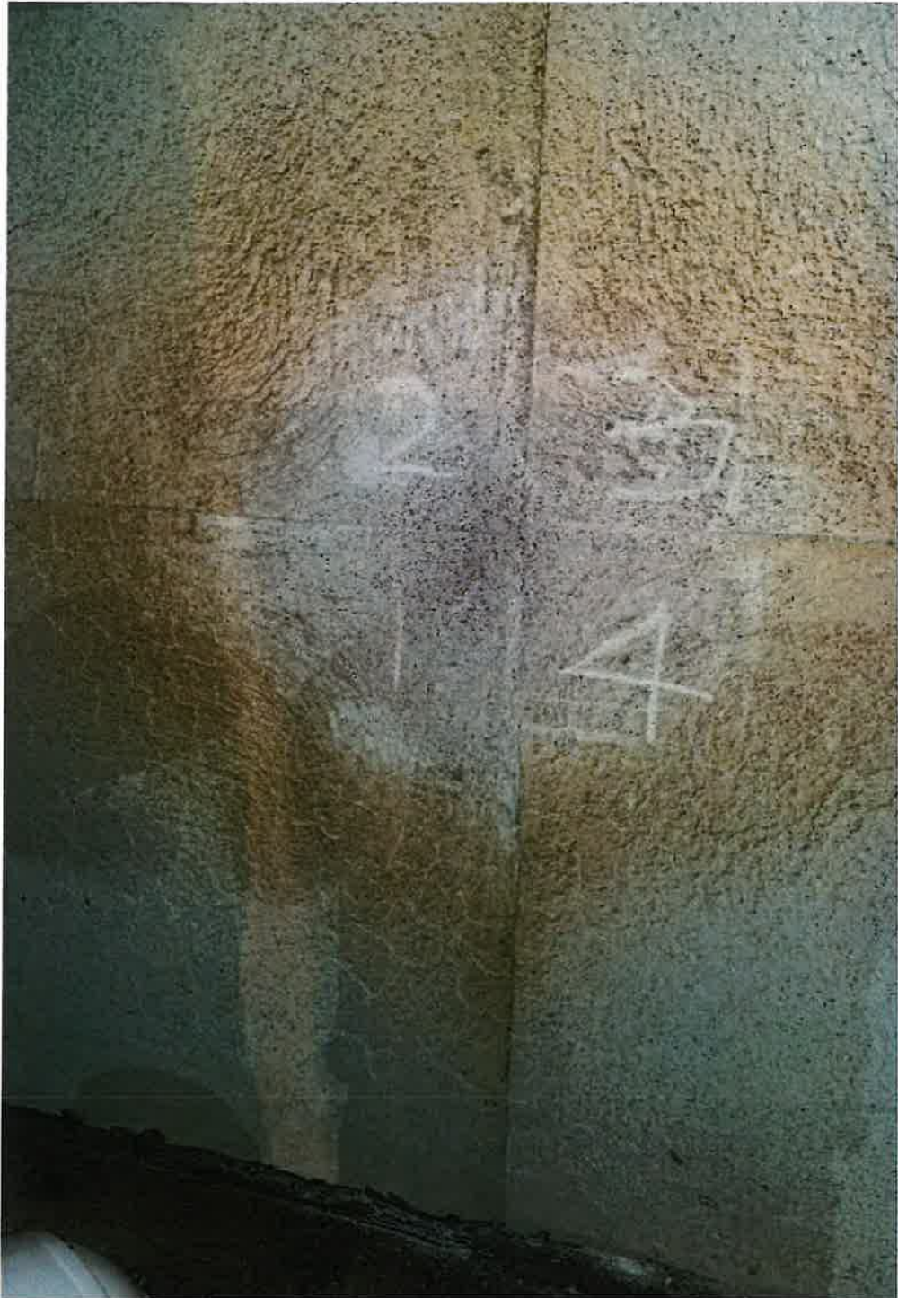
Figure 11 Close up showing condition of exposed face after attaining the ambient condition on exposed face
